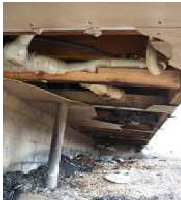
Underfloor damage caused by burning garden bed, suppressed by fire agency before it burnt into the house. Source: CSIRO
