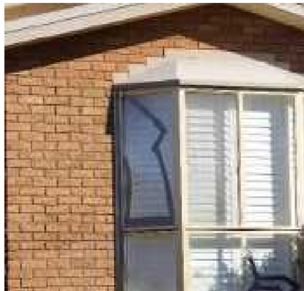
Cracked window from adjacent vegetation burning. Source: CSIRO
