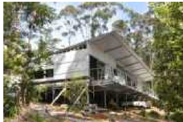
Bushfire resilient home under construction, using flame resistant sarking. Source: Ian Weir
