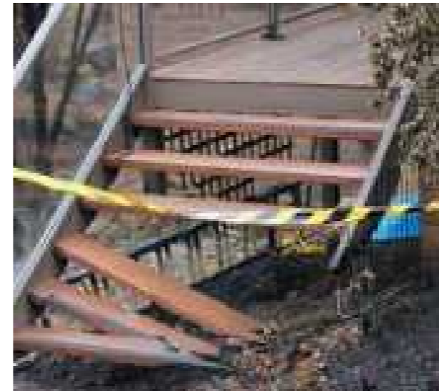
Potential issue with exit path on fire damaged stairs. Source: CSIRO
