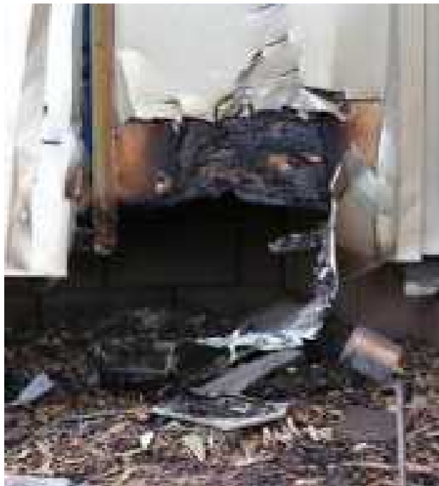
Damaged wall from burning vegetation. Source: CSIRO
