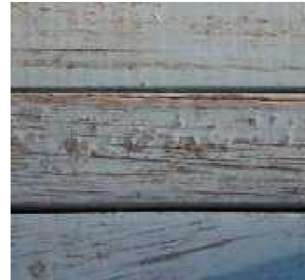
Damaged deck is vulnerable to ember attack. Source: CSIRO
