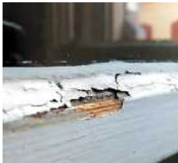
Damaged or decaying timber frames are vulnerable to ember attack.
