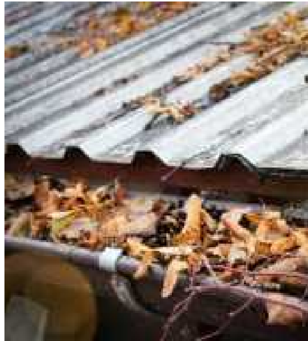
Debris accumulation in gutter.
